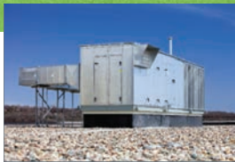
Air handling unit (A)
