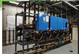
Parallel refrigeration rack (C)
